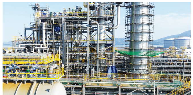
SNG Pipe Insulation
